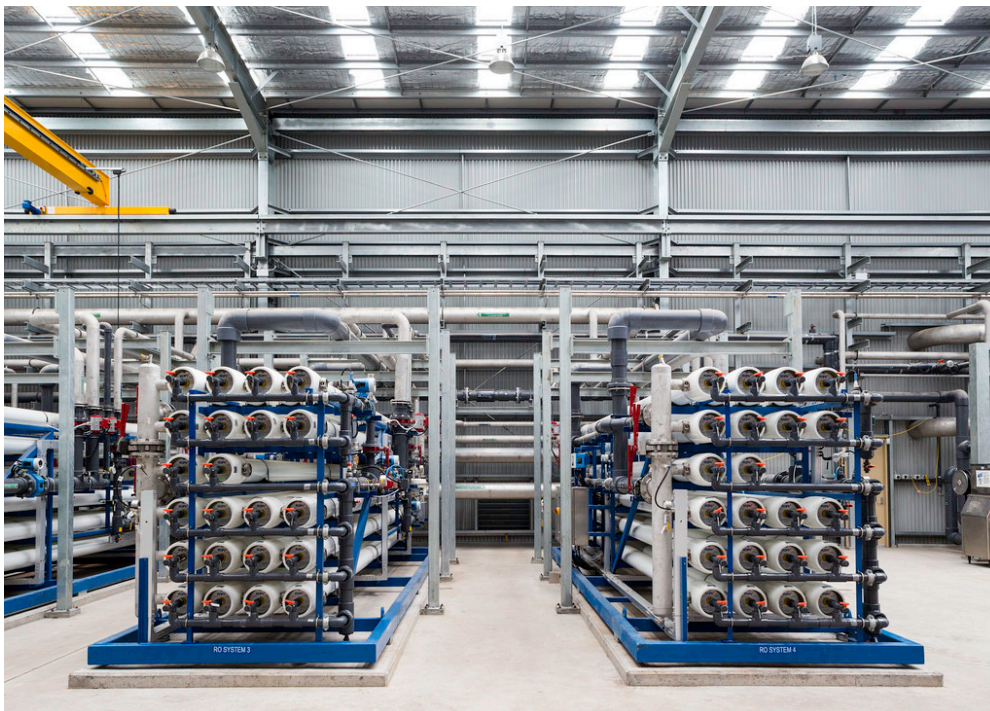
Image: Reverse osmosis trains, Kooragang Industrial Water Scheme
