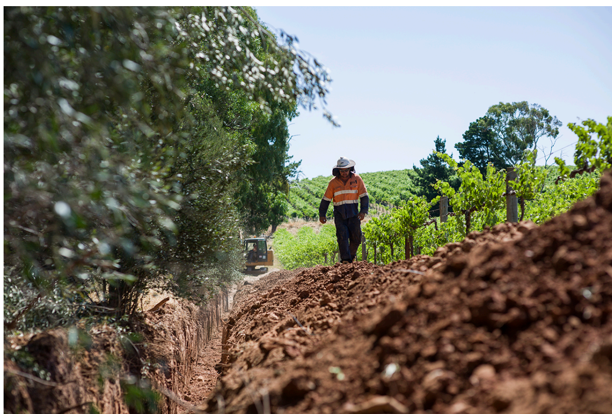
Image: An employee of WUA supplier CB&S Civil inspects a trench, Willunga Basin Water
